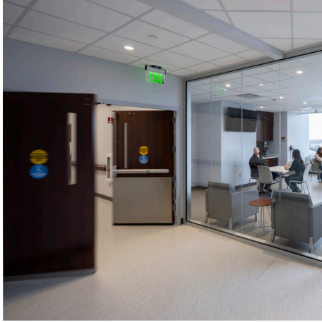
Von Duprin panic hardware provides code-compliant, intuitive egress with a simple push or lean, from Altru Hospital staff carrying equipment to patients with limited mobility.
